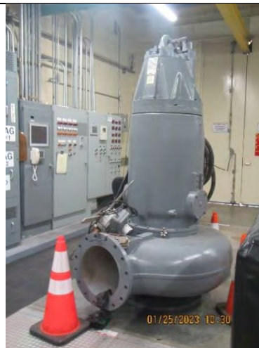
Photo 4: Spare pump for the D.A. Porath Pump Station located in the control room.
