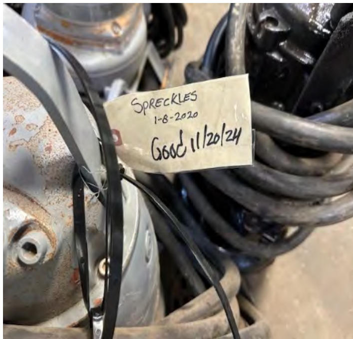
Photo 6: Corp Yard inspection (critical spare parts).
