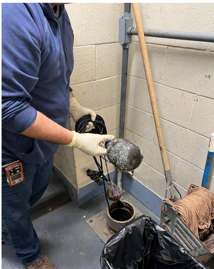
SITE B (Photo 8): View of float elevated by operator for simulated alarm test.
