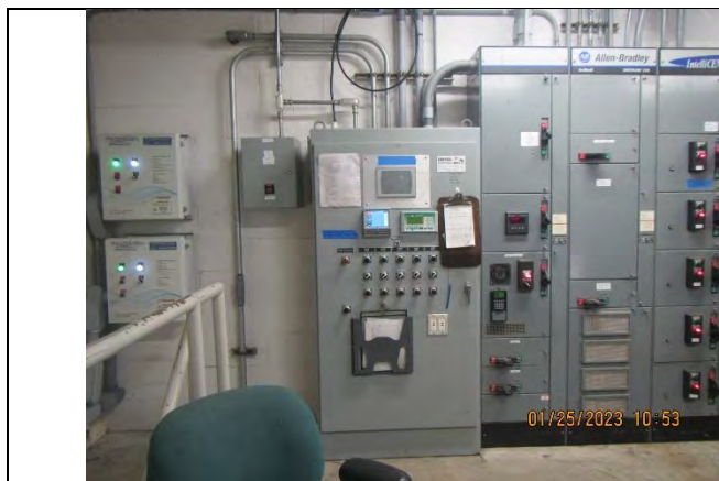
Photo 6: Electric grinder controls (left side of photo) in the control room of the Moran Pump Station.
