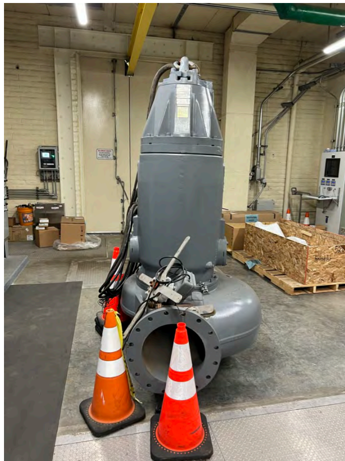
SITE A4 (Photo 6): Inspection of Flygt backup pump in readiness state at station.
