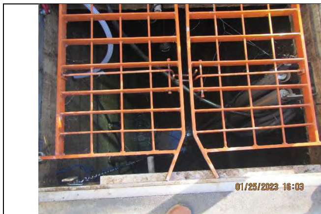
Photo 26: Safety gate over wet well at the Rodeo Pump Station. Minimal FOG observed.
