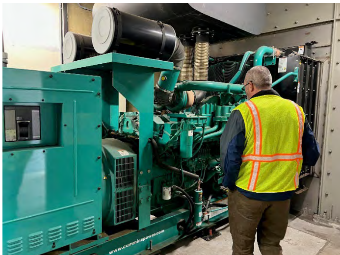
SITE C (Photo 5): Inspection of backup generator (Cummins model QST30-G5, rated at 1000 KWe 6 ).
