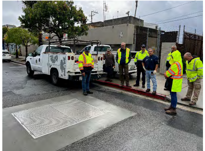
SITE C (Photo 2): Force main valve box array location.
