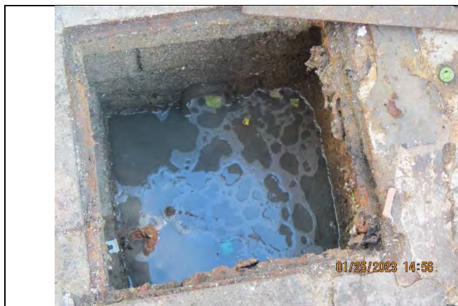
Photo 19: Storm drain located outside, in the back of Capitola Diner.
