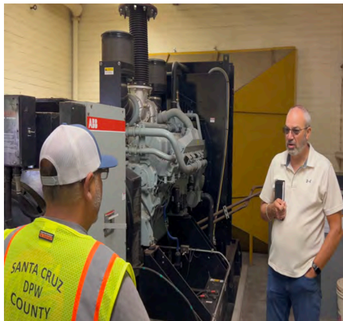
SITE A4 (Photo 2): Inspection of dedicated onsite diesel backup generator for station (view 2)
