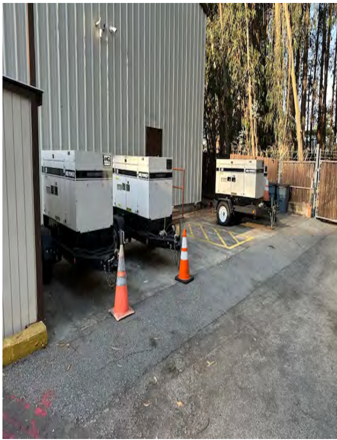
Photo 17: Corp Yard inspection (portable generators)
