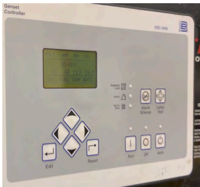
SITE A4 (Photo 4): Inspection of dedicated onsite diesel backup generator operator control panel; battery tender used on generator battery; digital gauge level on panel read "0" for oil and fuel, however day tank control panel levels read "full."
