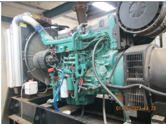
Photo 17: Generator at the Capitola Pump Station.
