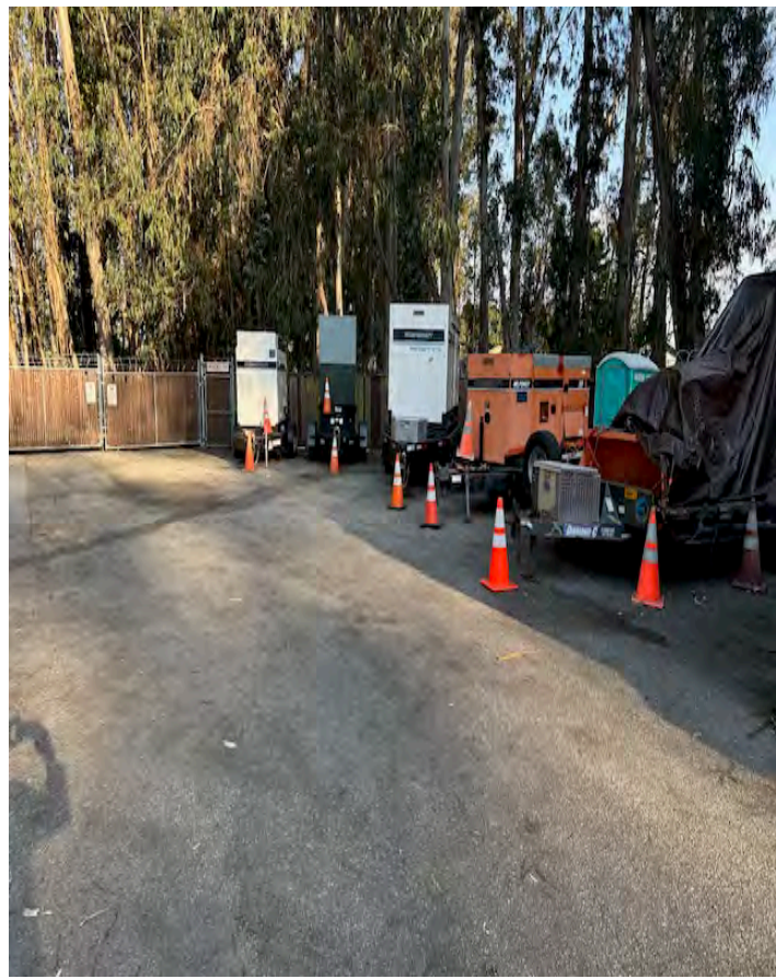
Photo 18: Corp Yard inspection (portable generators)
