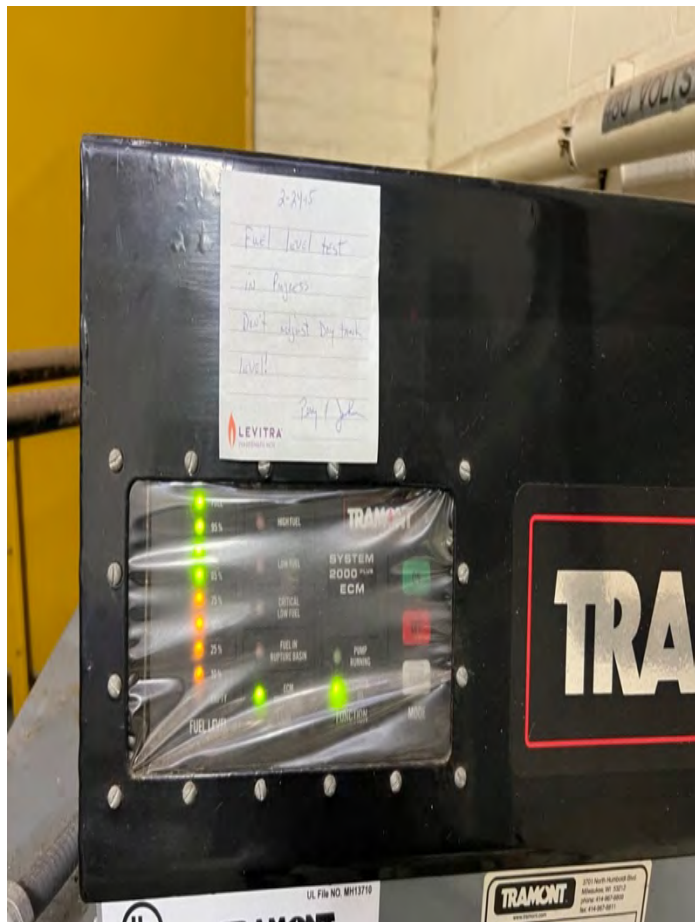
SITE A4 (Photo 5): Inspection of day tank generator fuel control station with fuel level observed at full capacity.
