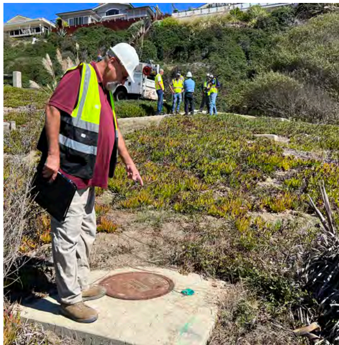
SITE B1 (Photo 7): View of maintenance manholes installed on beach looking east.
