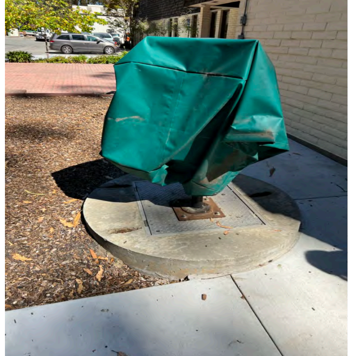
SITE A4 (Photo 10): Inspection of station bypass valve; the valve was observed in full-open position; District is aware of the issue and currently in design on a new project to replace valve and upgrade bypass capabilities.
