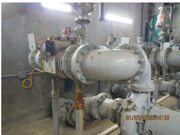
Photo 13: Old pumps at the Capitola Pump Station.
