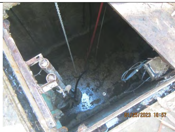
Photo 7: Wet well of the Moran Pump Station with a visible FOG mat and rusted/corroded components.
