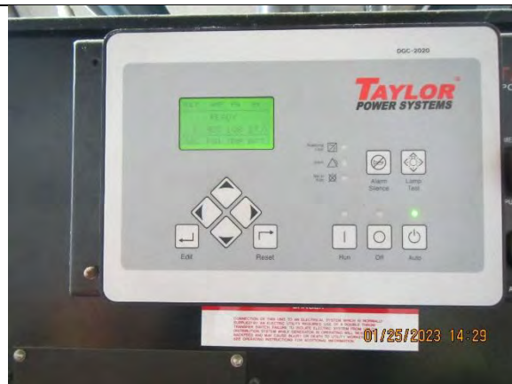
Photo 18: Screen on generator showing 92% fuel level at the Capitola Pump Station.
