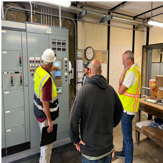
SITE B1 (Photo 8): Inspection of motor control center (MCC) and interviews with field operations staff.
