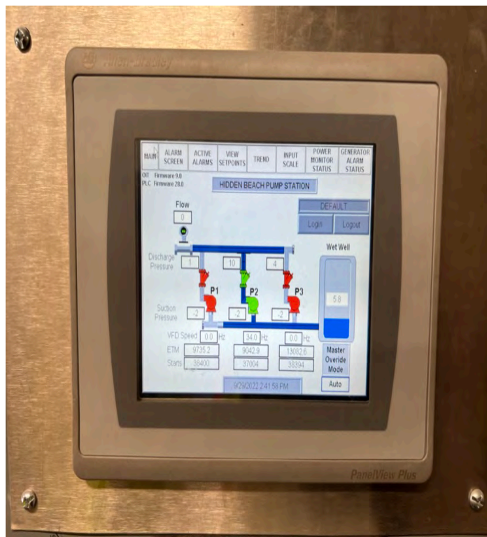
SITE B1 (Photo 11): Inspection of station alarm panel (view 1).
