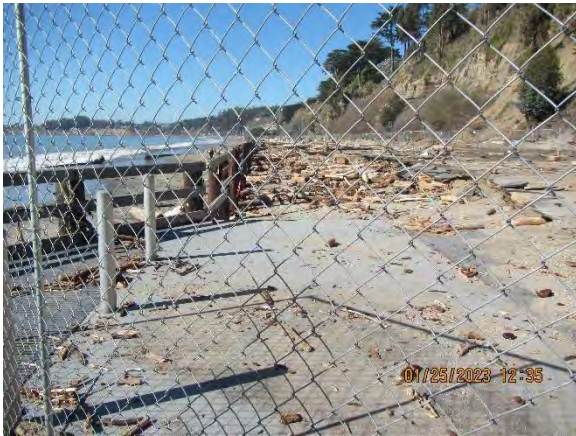
Photo 11: Parking lot and walkway at the A1 Pump Station, destroyed by the recent storms.
