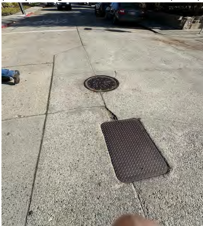
Photo 29: Inspection of 36-Inch Force Main (Valve and crossover line to allows portions of the FM sewage to divert to the gravity system)
