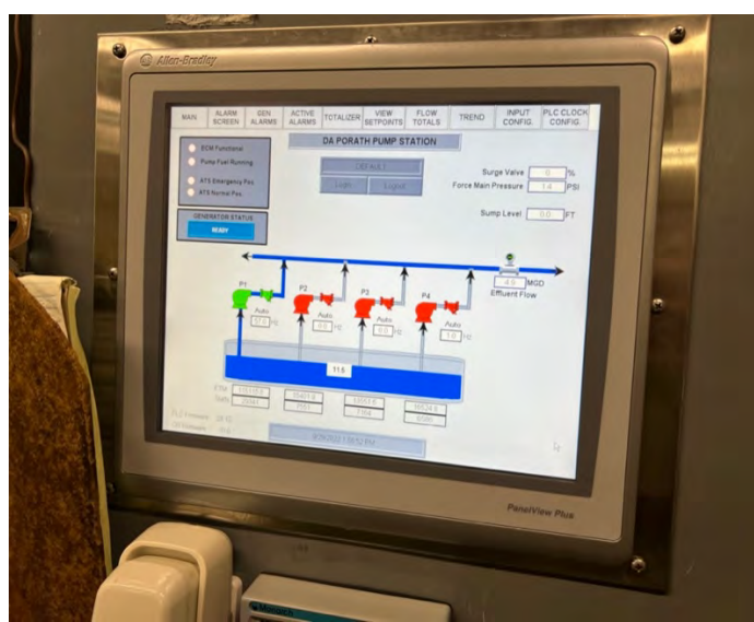
SITE A4 (Photo 8): Inspection of operator motor control panel on MCC; all pumps in readiness state.
