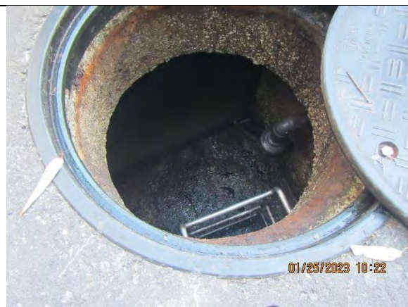
Photo 2: Manhole upstream of the D.A. Porath Pump Station with an observed wet bench.
