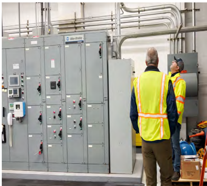
SITE B (Photo 5): View of motor control center (MCC).
