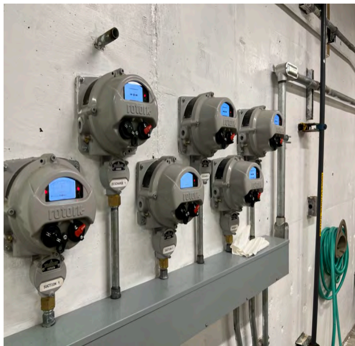
SITE B1 (Photo 13): Inspection of electronic valve controls.
