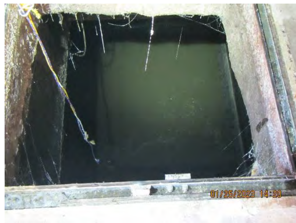
Photo 16: Wet well at Capitola Pump Station with some cobwebs and minimal FOG.
