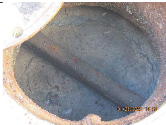
Photo 20: Grease interceptor for the Capitola Diner with a visible high solids content.
