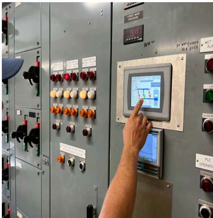
SITE B1 (Photo 10): Station SCADA system control screen.
