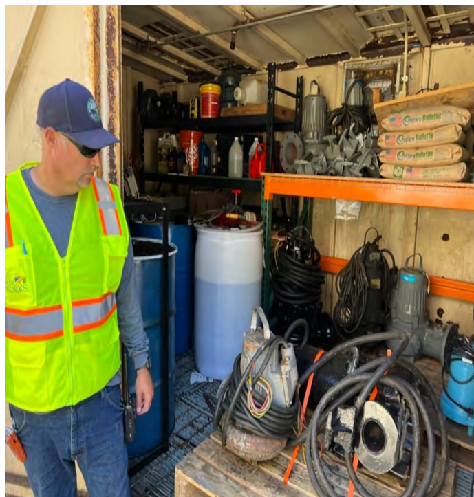
SITE A3 (Photo 4): Inspection of system spare parts and equipment.
