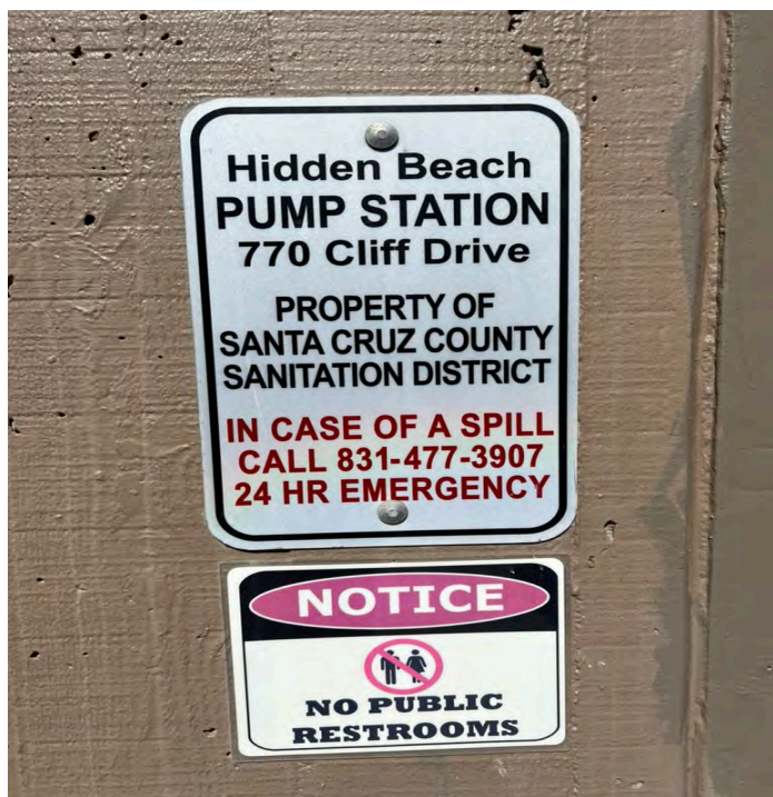
SITE B (Photo 5): View of pump station emergency notification signage.
