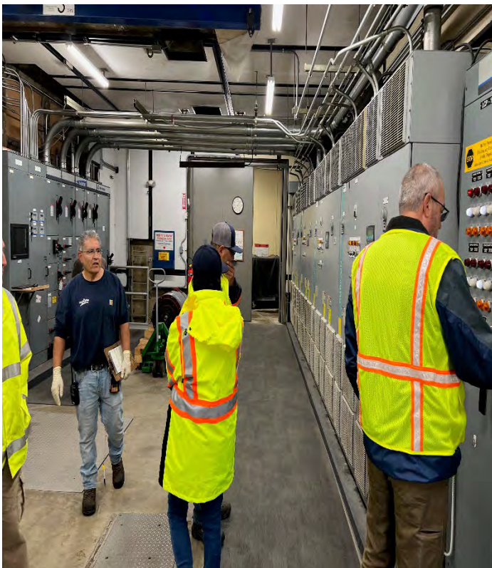
SITE C (Photo 3): Inspection of station controls and motor control center (MCC).
