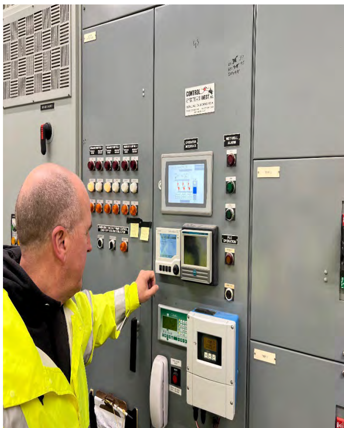
SITE B (Photo 7): Inspection of operator controls at station; a successful "simulated high float" alarm test was conducted by station operator.
