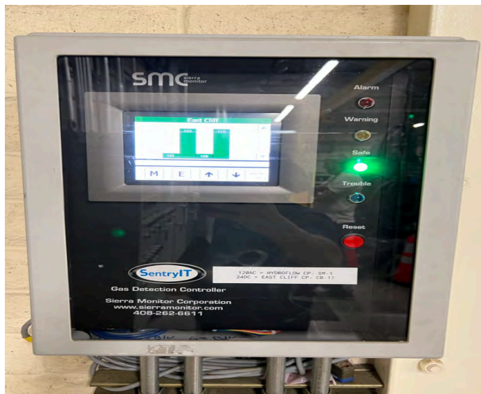
SITE A4 (Photo 7): Inspection of hazardous gas detection control panel inside station.
