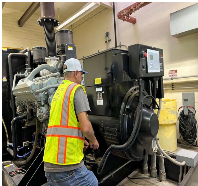
SITE A4 (Photo 1): Inspection of dedicated onsite diesel backup generator for station (view 1); field staff were not comfortable simulating readiness scenario for failed power failure, so simulation was not conducted during inspection.
