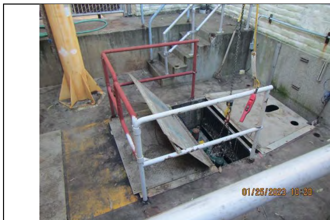
Photo 1: Crane attached to the grinders at the D.A. Porath Pump Station.
