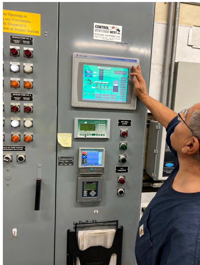
SITE C (Photo 7): Inspection of station controls/motor control center (MCC) with station operator.
