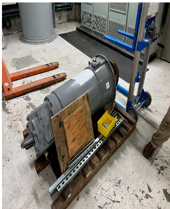
SITE D (Photo 6): Inspection of Flygt backup pump in readiness state at station.
