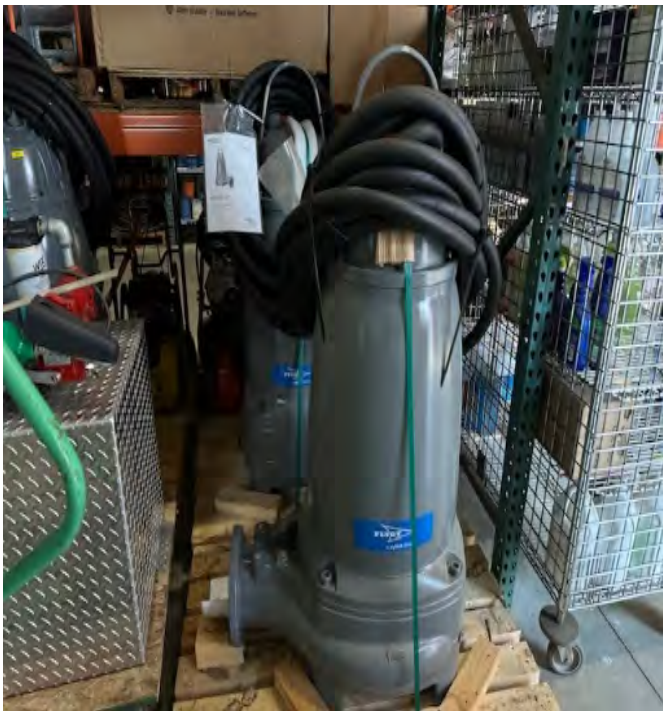
Photo 3: Corp Yard inspection (critical spare parts); Spare Pumps all are labeled for the station and are compatible for most stations ( Best Practice).
