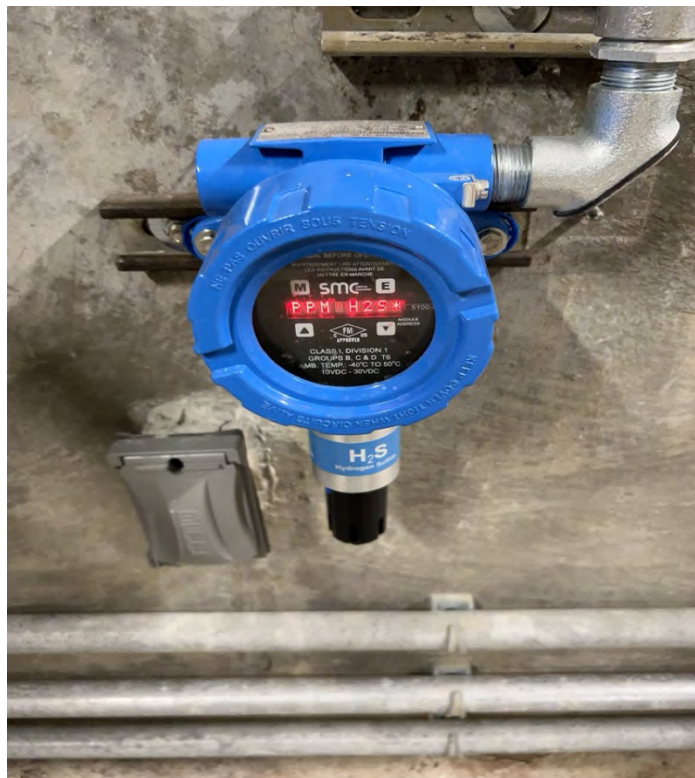
SITE B1 (Photo 15): Inspection of station hazardous gas monitor.
