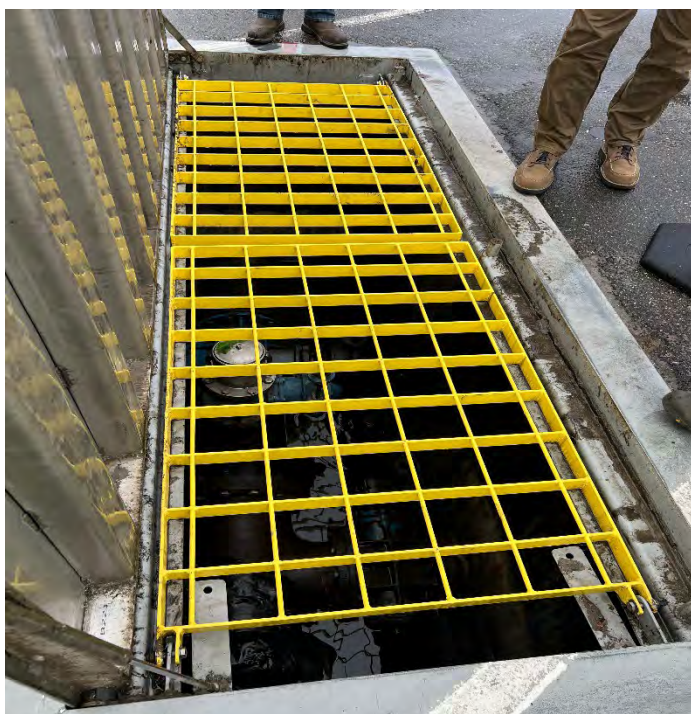
SITE B (Photo 4): View inside force main/bypass connection manifold vault.
