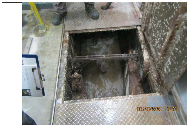
Photo 8: High flow in channel leading to the wet well of the Hidden Beach Pump Station.
