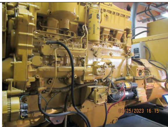
Photo 27: Generator at the Rodeo Pump Station observed to be in great condition
