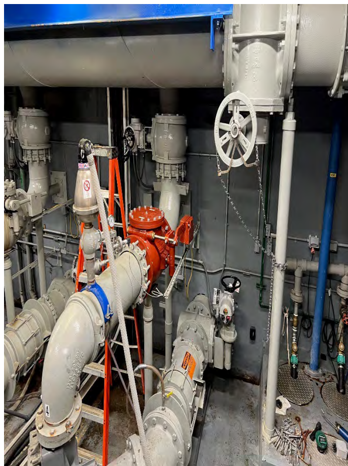
SITE C (Photo 8): Inspection of pumps/valves/force main; one gate valve auto system was observed out of service (operators currently manually open/close valve, 80 turns).
