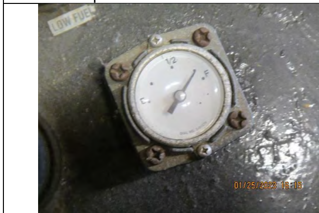
Photo 28: Fuel level on generator indicating approximately 75% full.
