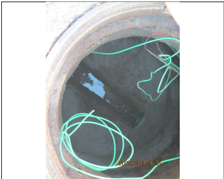
Photo 29: Manhole near the East Cliff replacement project with exposed wire.
