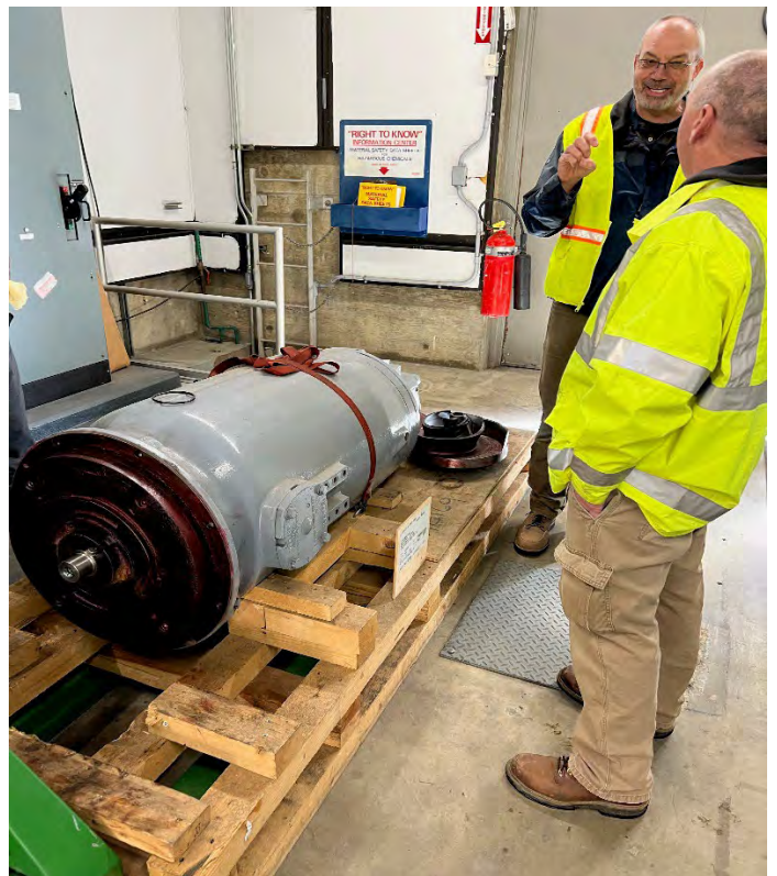
SITE C (Photo 4): Inspection of backup pump.
