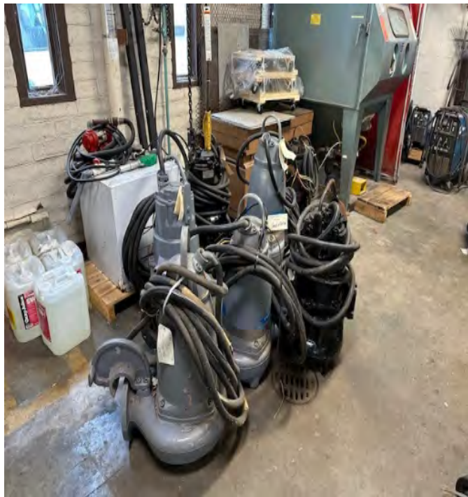
Photo 4: Corp Yard inspection (critical spare parts).
