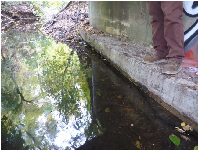
Photo 2 Footing Condition, Abutment 1
