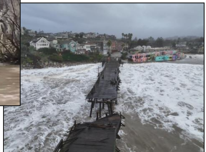
Right: Capitola Pier was damaged. Seacliff Pier was destroyed.
