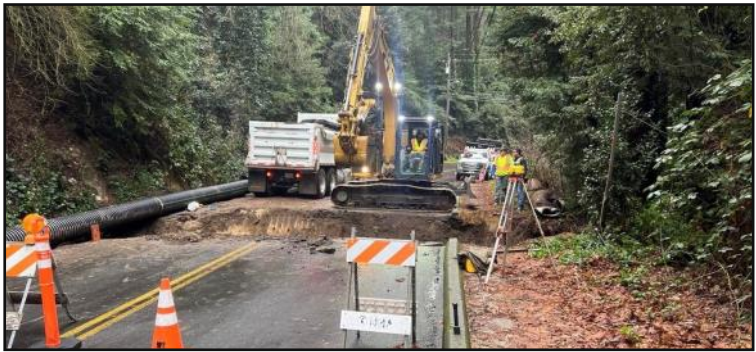
Storms left behind a new round of storm damage throughout the County. It will likely take several years to repair the local road network.
